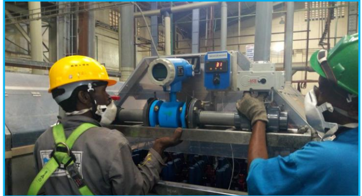
D&S Technicians on site as they install monitoring and control equipment for the factory's automated cooling system.
