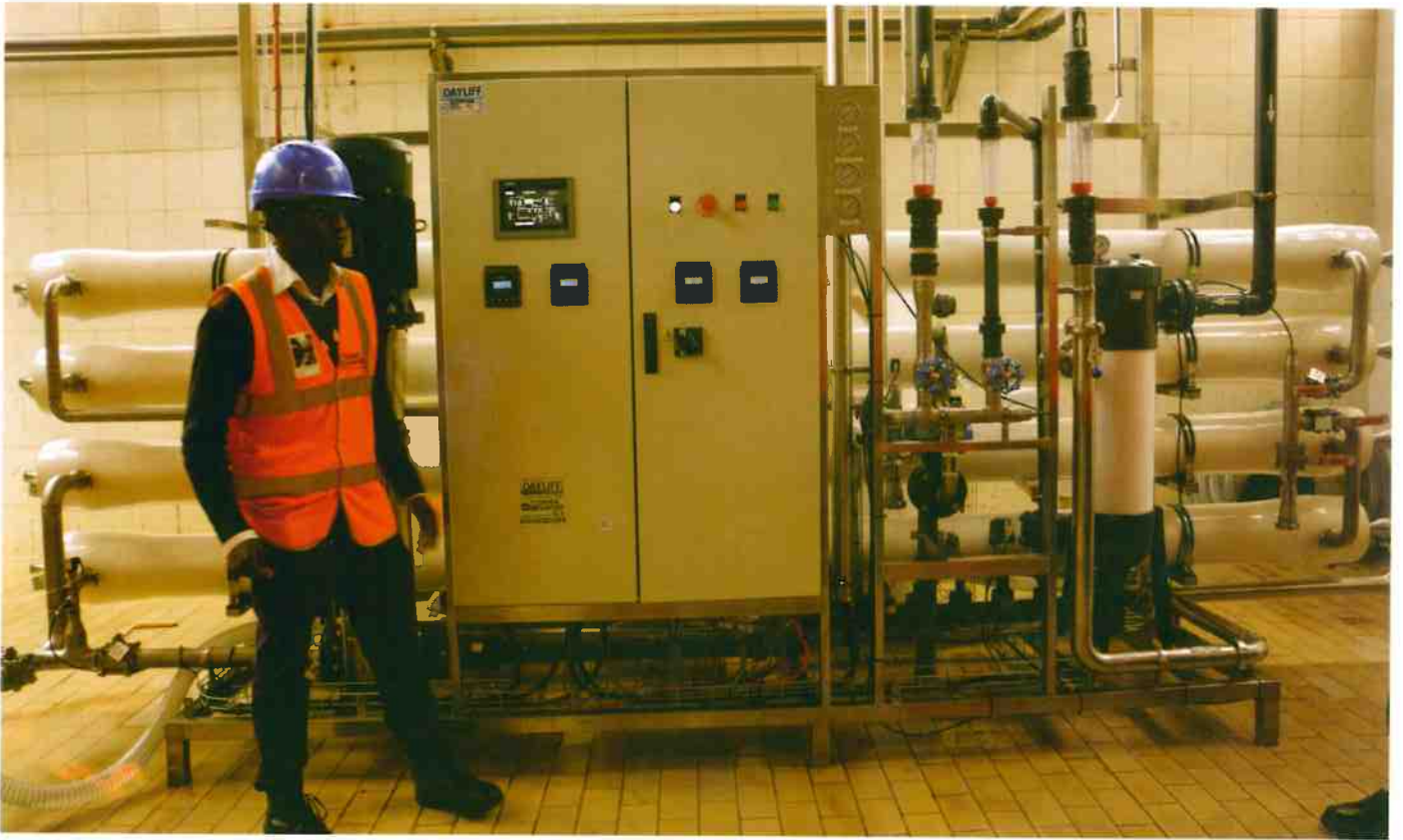
Davis & Shirtliff Technician inspecting a Dayliff Reverse Osmosis Plant.
