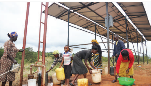
Dayliff remote monitoring solar powered borehole pump installed at Mwala
